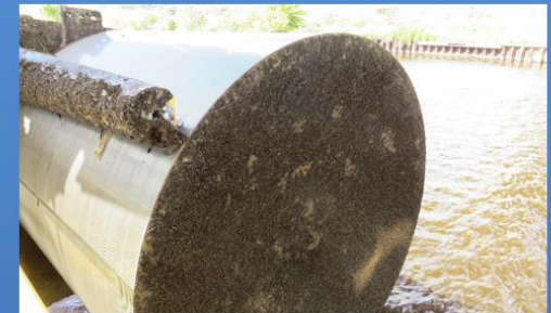
Valley Power Plant, Milwaukee, WI
